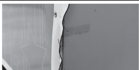
Other's riveted construction with damage
